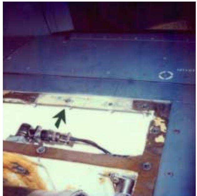
Arrow indicates location of cracks
