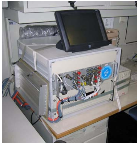
Figure 8 Data Acquisition Unit (DAU), installed in the vicinity of the wheel house.
