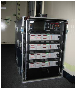
Figure 25 Telemetry receivers and signal combiner installed used by the test centre.
