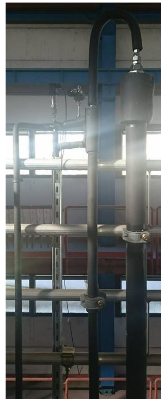
Figure II.4 – Gas separator (a) scheme (red circle: gas; blue hexagon: water) and (b) installed at the flow loop.
