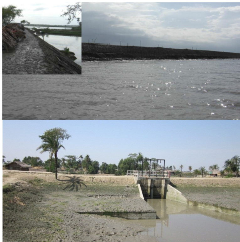
Figure S3: Photograph of a typical polder, earthen embankment, above, source: (Ortega, 2009), and a sluice gate structure of a polder in Dacope - a coastal area in Bangladesh. These are typical of other Asian deltas. In Bangladesh alone, 123 polders, including 49 sea-facing polders, were constructed in the 1960s to protect low-lying coastal areas from tidal floods and saline intrusion (The World Bank Group, 2010).
