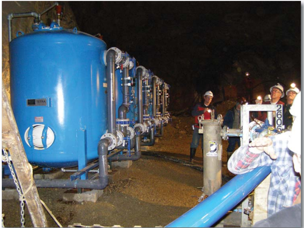
Water treatment plant at the Drumlummon Gold/Silver Mine.
