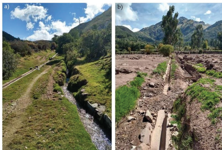
Figure 6. (a) A modern concrete canal with control gates adjacent to an earthen canal. (b) Destruction to concrete canal following March 2019 debris flow.
