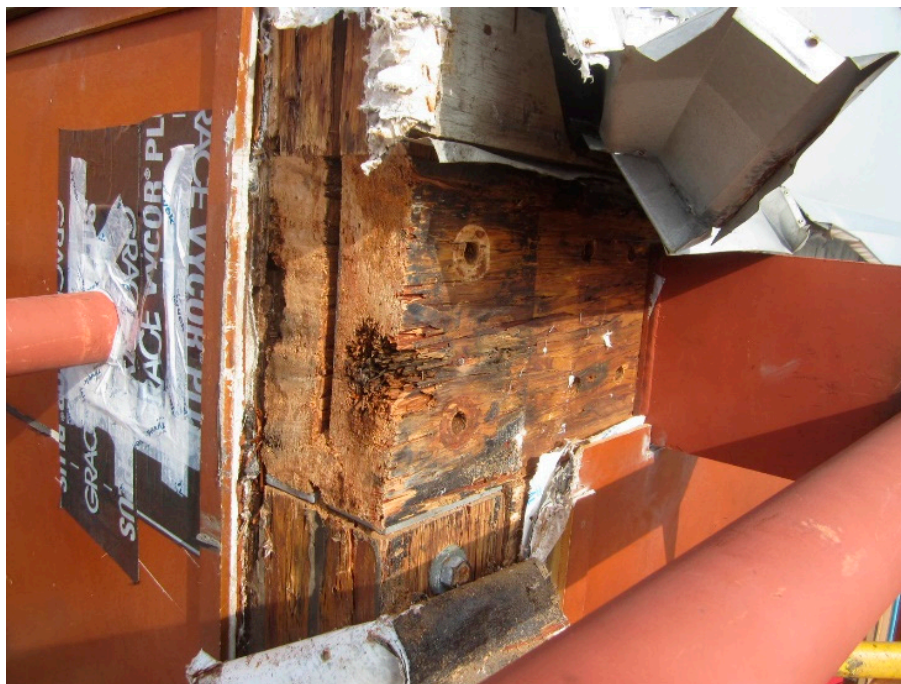
Figure 6. Moisture ingress and decay in a typical engineered wood structural member. Photo: Wiss Janney Elstner, Inc.
