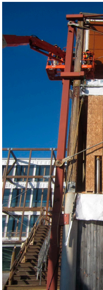
Figure 5. Engineered wood structural members expressed on the exterior envelope of the building. Photo: Wiss Janney Elstner, Inc.
