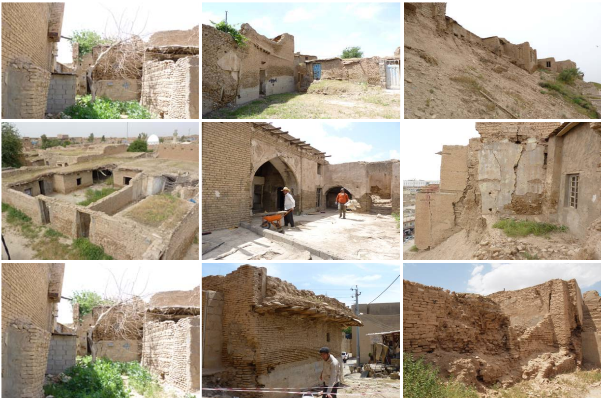
Partially collapsed structures
