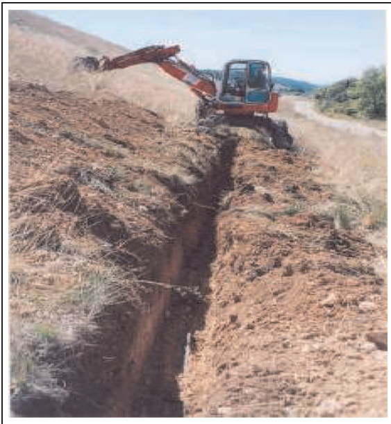
Figure 5. Digging up of the trench for optical fiber installation along the dike.
