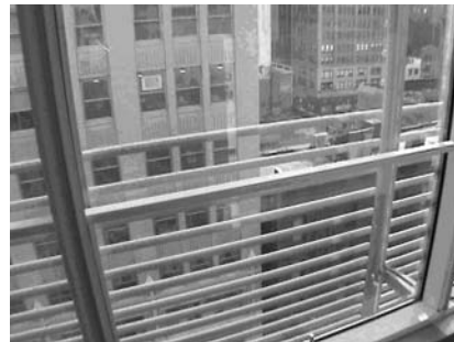
Fig 8. Spacing of the CRF in the lower portion of the office window.
