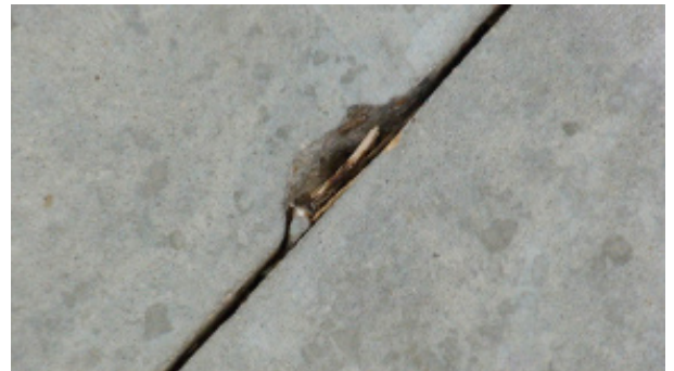
FIGURE 5.35: Concrete can be damaged at its edges, but can also be inexpensively patched.
