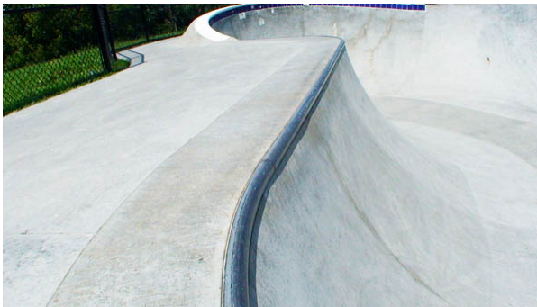
FIGURE 2.18: Round steel coping in the bowl at the Kansas City Skate Plaza.
