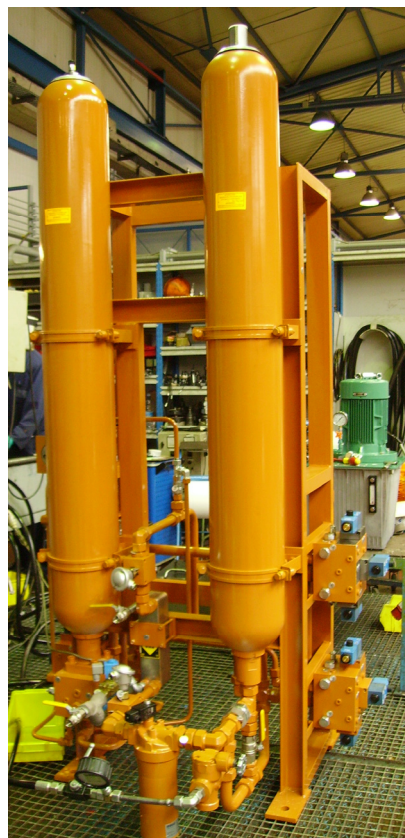
Figure 7. HP and LP accumulators.
