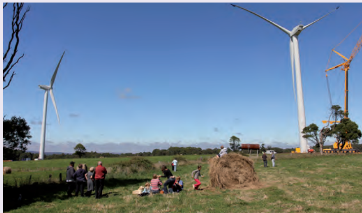
Local members watch final stages of construction, March 2011. Image provided by Tibor Hegedis.
