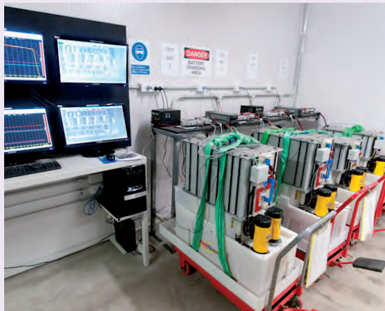
A row of freshly manufactured RedFlow batteries undergoing testing before shipment to customers in June 2011. Image provided by RedFlow Ltd.
