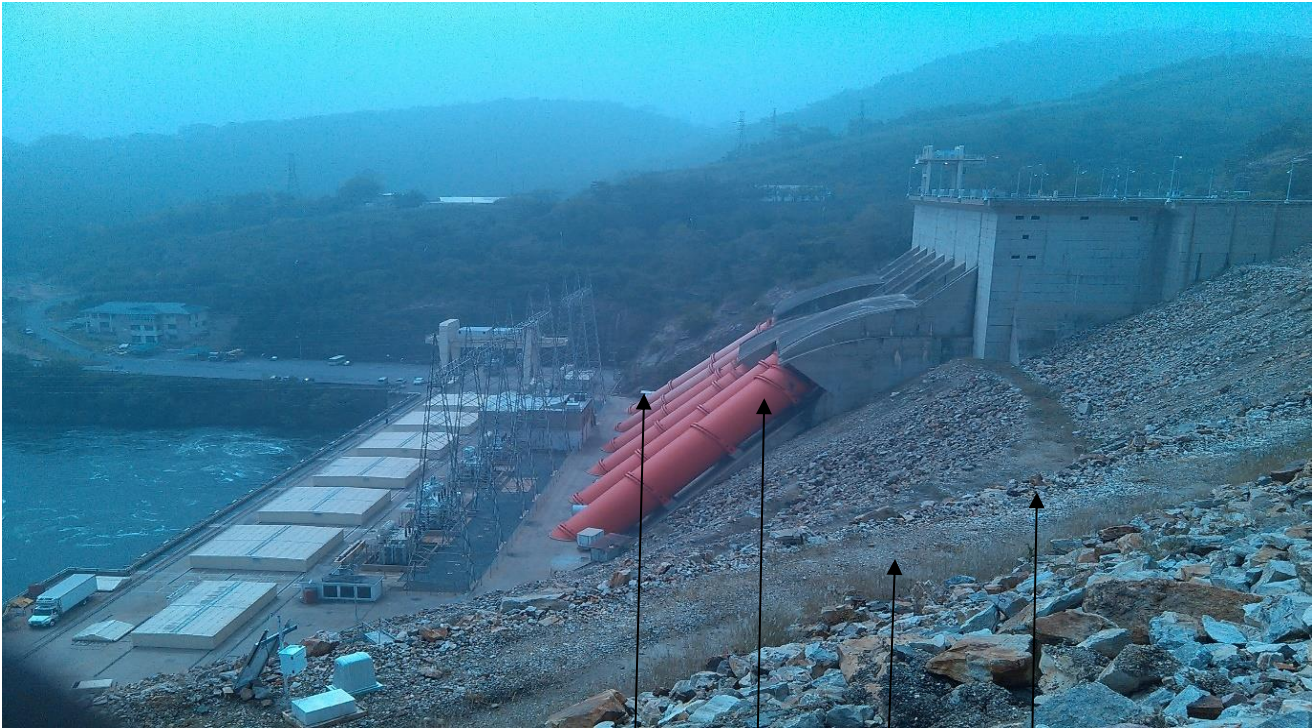
Figure 16: Observed climate related effects on some portions of the Akosombo dam. Source: Author, 2021
