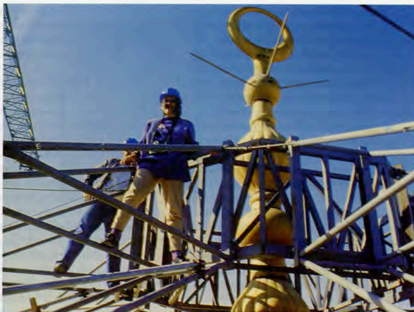
Above: Beatrice St. Laurent on the scaffolding at the top of the Dome of the Rock, at the beginning of King Hussein of Jordan's second major restoration project in 1993. Also in the photograph is the Palestinian Chief Engineer in charge of the project. The process of removal of the old anodized aluminum panels had just begun.
