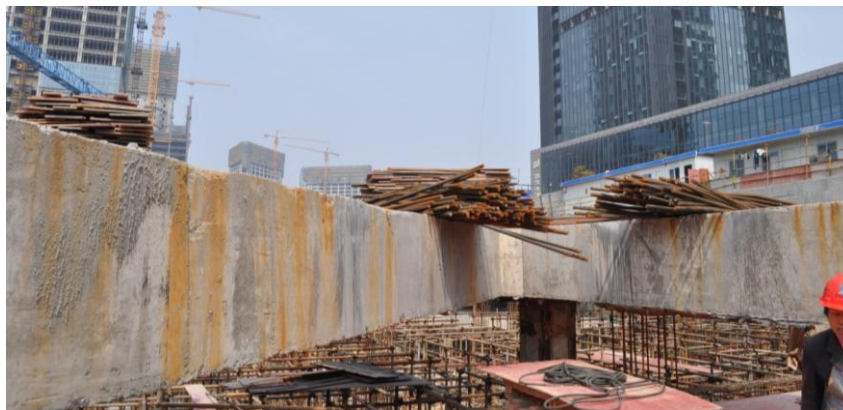
Figure 10.2 Inappropriate storage of rebar at Project B
