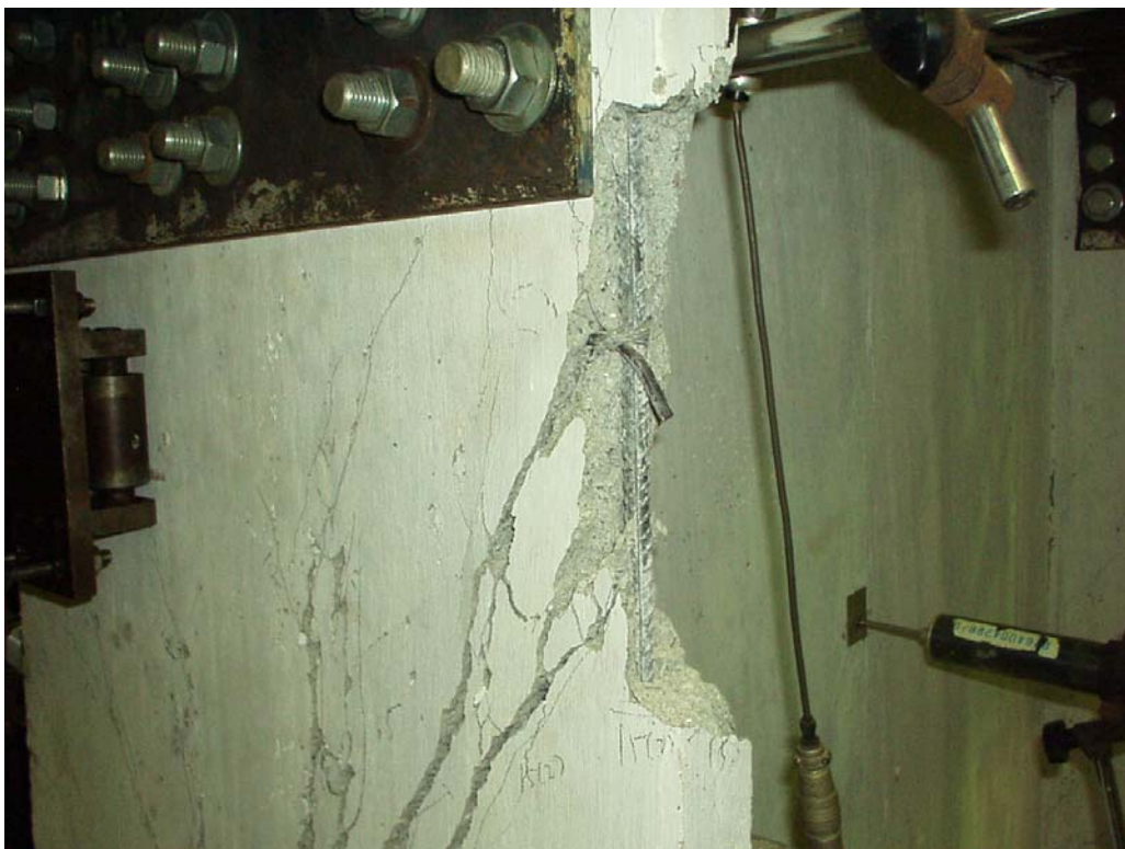
Figure 4.31 Spalling concrete of the upper right part of the right flange wall
