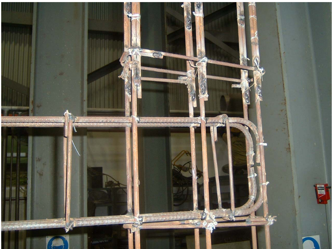
Figure 2.7 3D view of the lap splice of columns above the 1 st story joints
