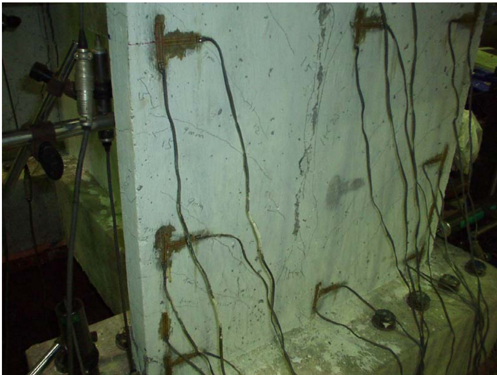
Figure 4.33 Shear cracks on the left flange wall
