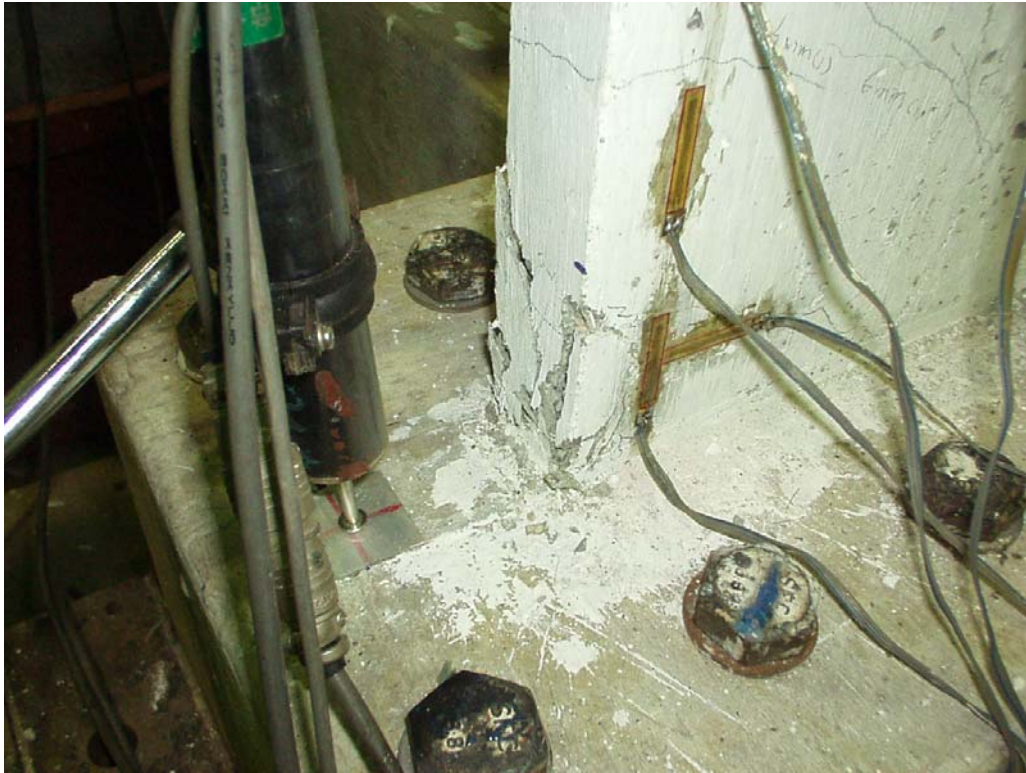
Figure 4.34 Spalling of the left flange wall corner
