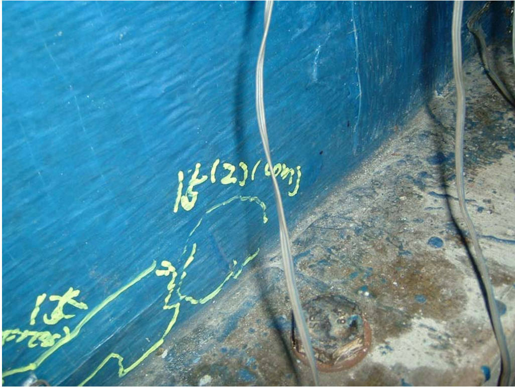
Figure 4.38 FRP debonding of the right flange wall (the second 15 mm cycle)
