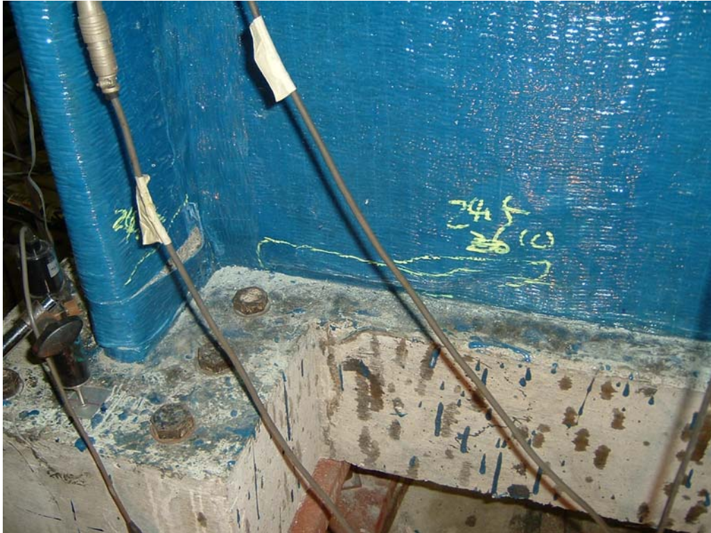
Figure 4.42 Crushing of the right flange wall corner at 24 mm top displacement
