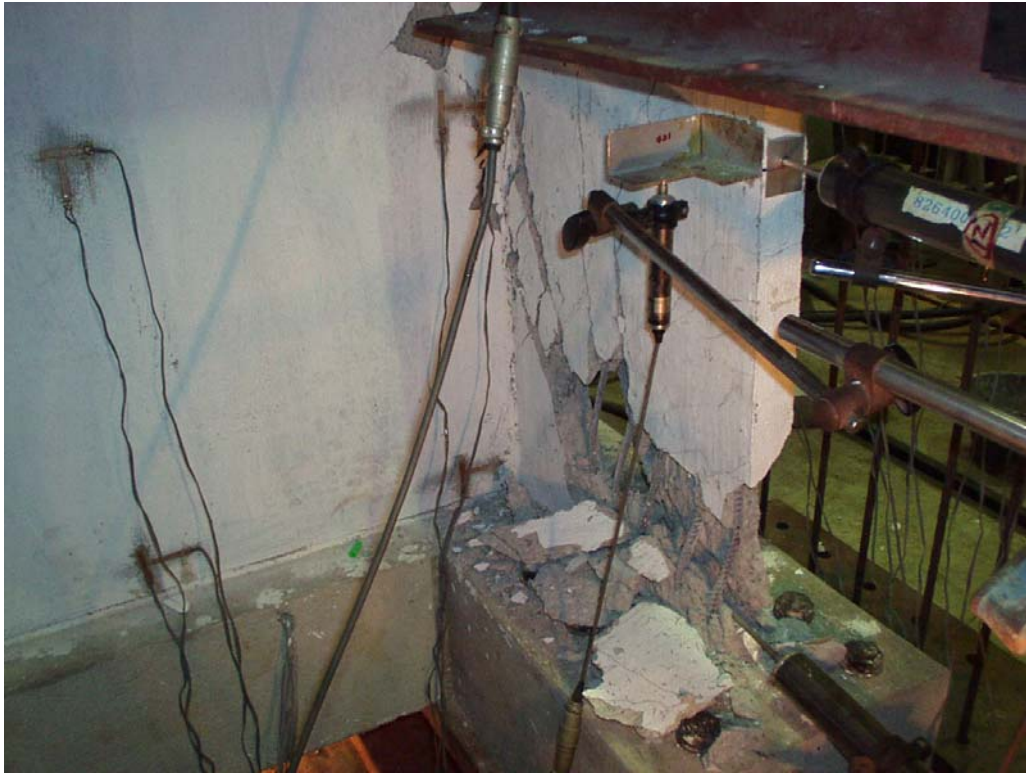
Figure 4.32 Spalling of concrete of the bottom part of the right flange wall
