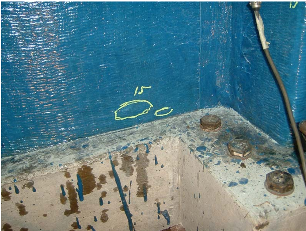
Figure 4.37 First FRP debonding of the web wall
