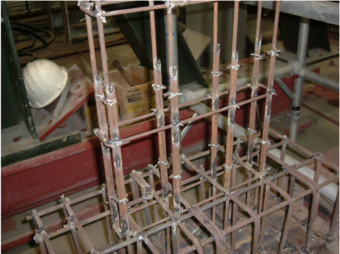
Figure 2.6 3D view of the lap splice of columns above the base block
