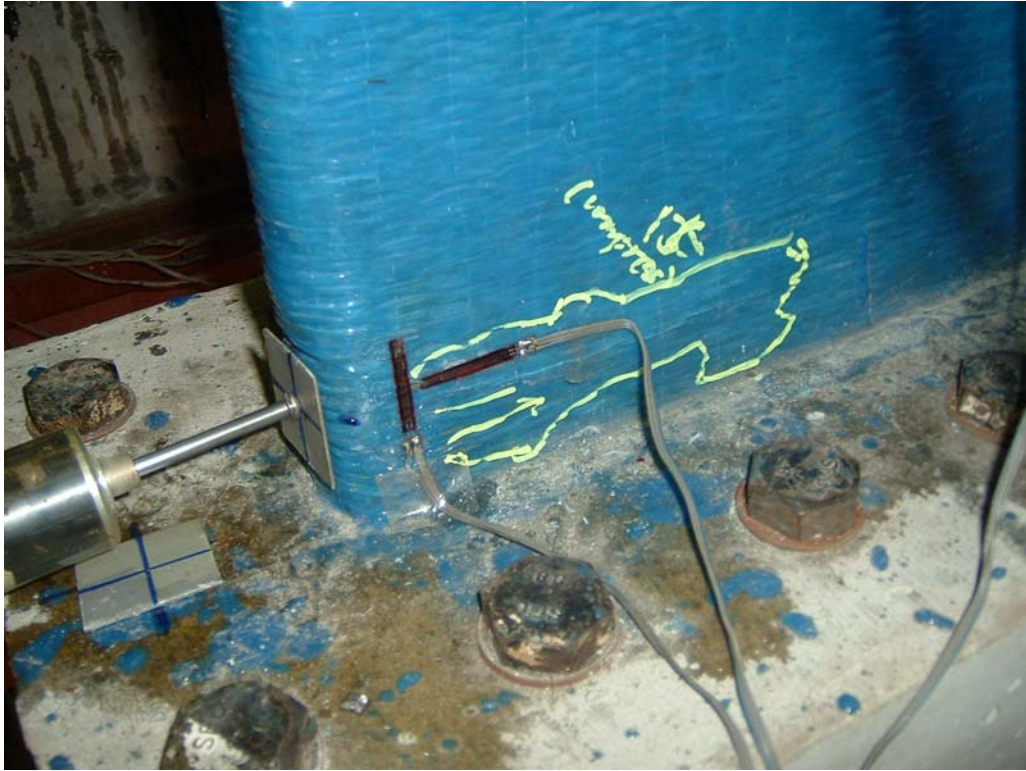
Figure 4.36 First FRP debonding of the right flange wall
