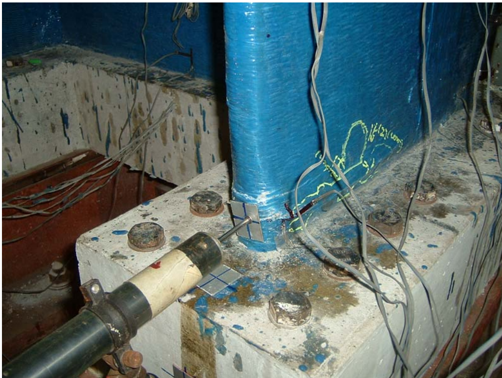
Figure 4.39 Crushing of the corner of the right flange wall at 16 mm top displacement
