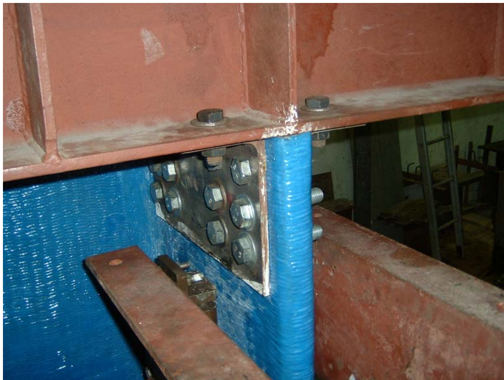
Figure 4.19 3D view of connections of U beams to L angles and L angles to walls
