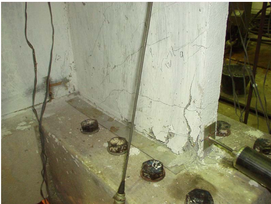
Figure 4.29 First spalling of the concrete of the right flange wall
