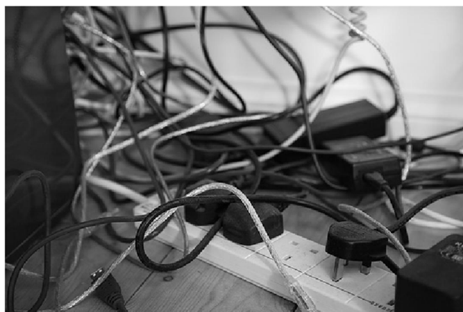
Figure 6.14: Tangled mess of power cords and chargers
