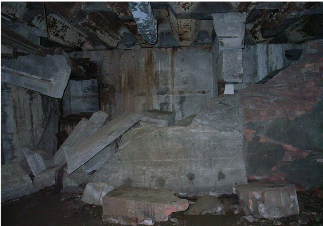
Illustration 84. Evidence of an explosion is everywhere. The walls separating the main room with the ante-chambers have collapsed. The crawl through leading to the escape ladder and the old 9.2 inch gun magazine 17m above can be seen on the left of the wall ahead. (Author)
