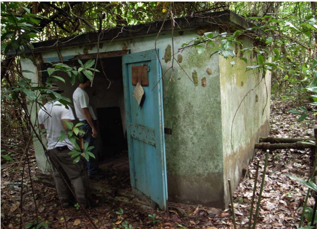
Illustration 43. Pump room, located southwest of the water storage tank. (Aaron Kao)
