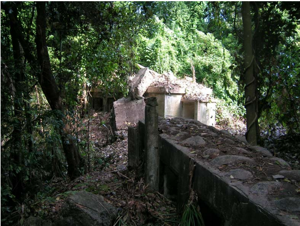
Illustration 63. The gunner's shelter revealed. The magnitude of the magazine explosion can be witnessed by the amount of concrete rubble and earth thrown up and almost burying the structure. (Author)
