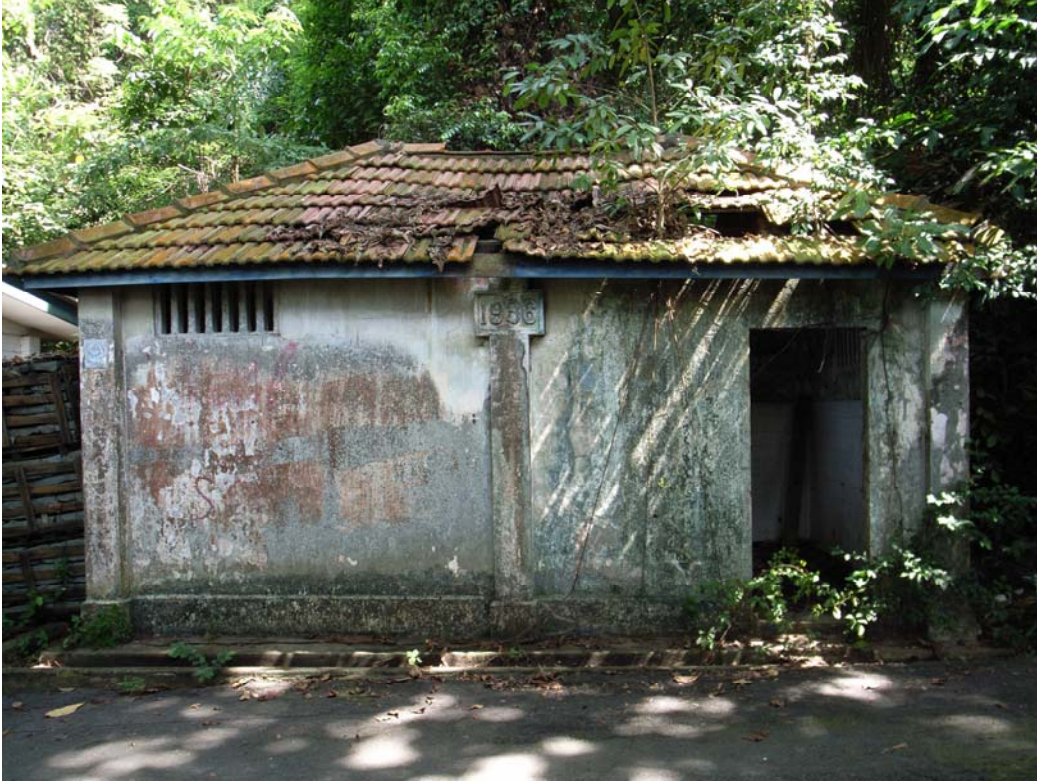
Illustration 78. The bathroom block comes next after the kitchen and barracks. (Aaron Kao)
