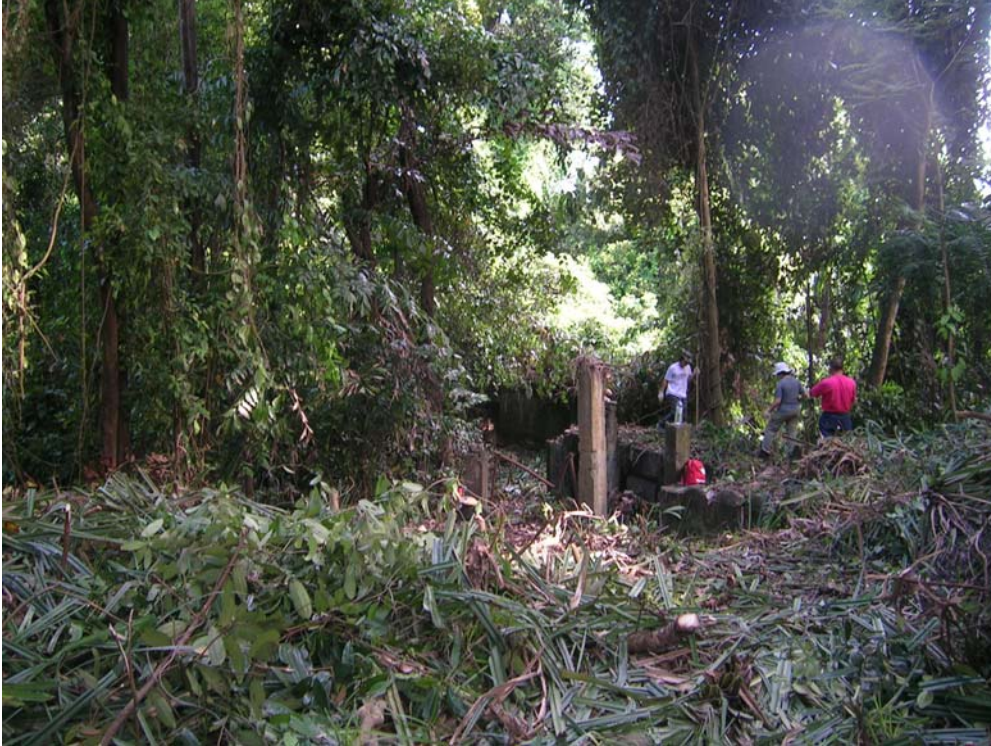
Illustration 54. Work barely began at the site of the 6 inch Gun No.2 emplacement. (Aaron Kao)
