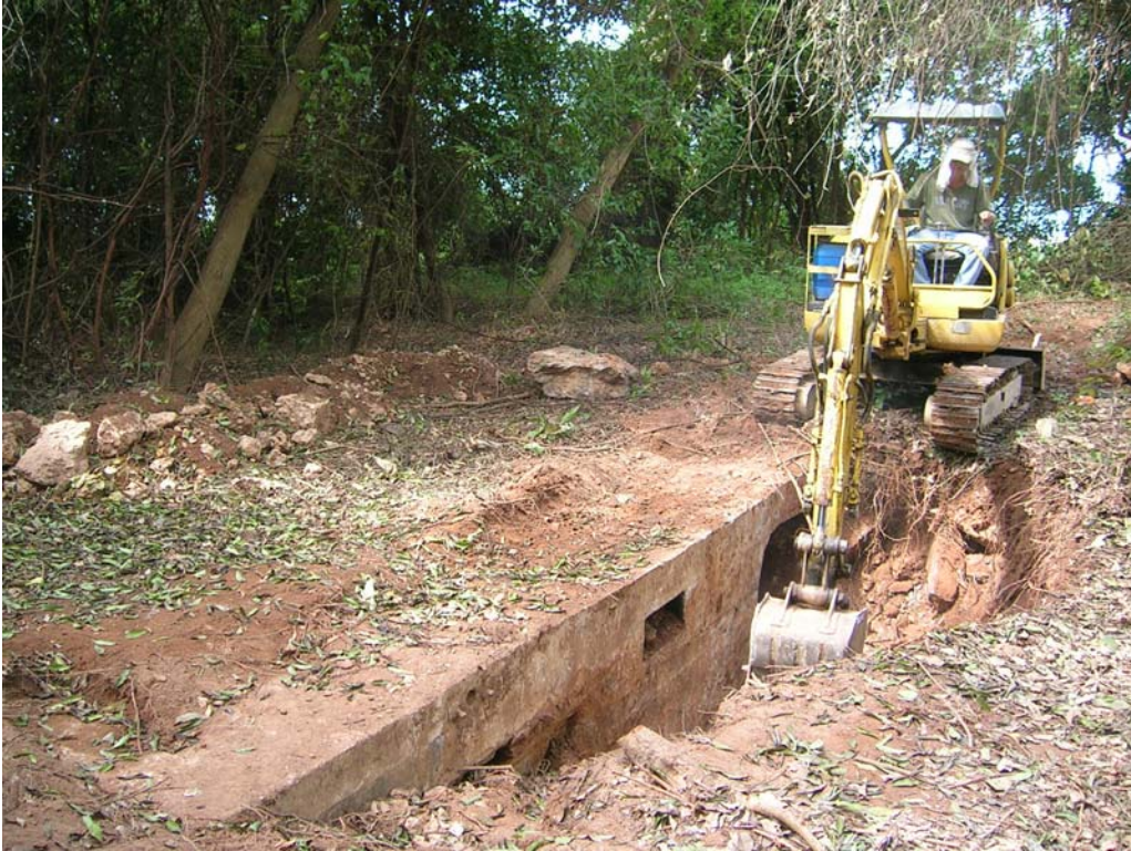
Illustration 24. Test trenching located the edge of the 9.2 inch Gun No.1 shell hoist and determined that the emplacement was covered by construction rubble fill with no artifacts allowing a mechanical excavator to be brought in for the excavation. The small rectangle recess (centre) is for the firing primers. (Author)
