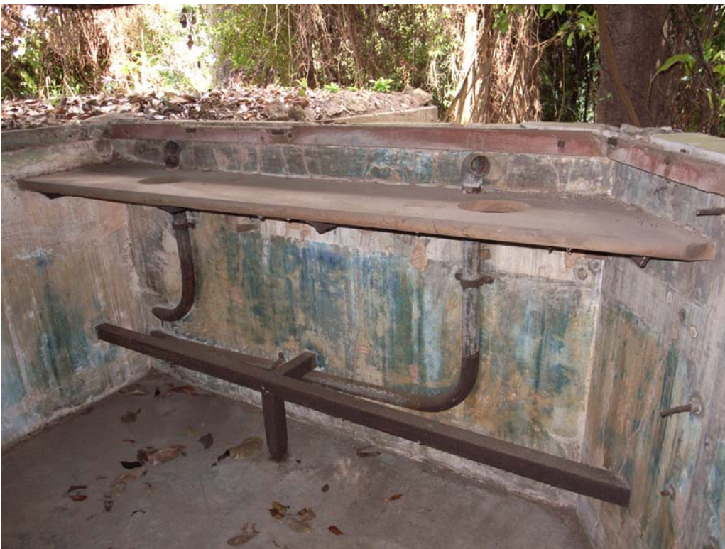
Illustration 73. Interior of the upper level. A timber bench with mild steel voice pipes connection to the lower BCP. (Aaron Kao)
