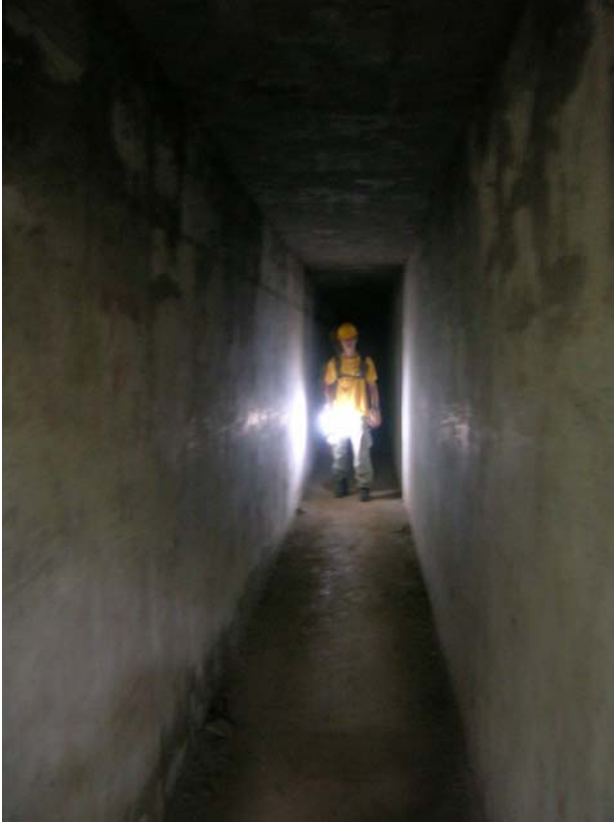
Illustration 87. The 31m long passageway leading into the Blakang Mati command centre in the northwestern slope of Mount Serapong. (Author)
