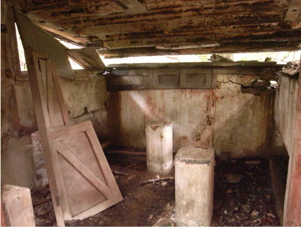
Illustration 22. Interior of PF Cell No.2. Note the pedestals for the position finding equipment are still in situ. (Aaron Kao)
