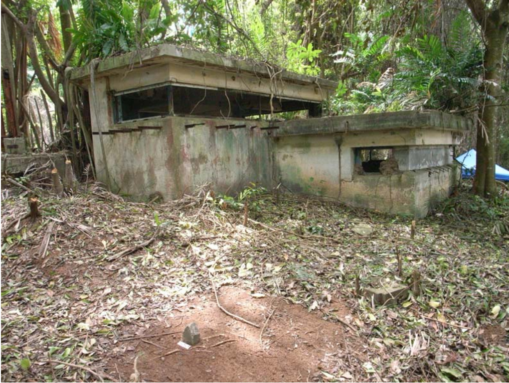
Illustration 80. Eastern view of Connaught's BCP. It too is a split leveled structure. (Aaron Kao)
