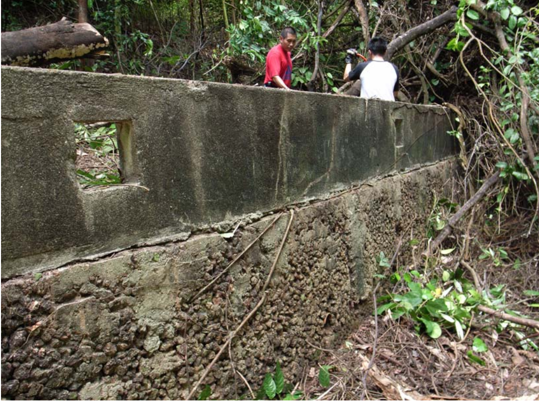
Illustration 38. Infantry Post No.5 along the western edge of the water catchment runoff was made up of a concrete wall with firing ports at every 2m distance. (Aaron Kao).
