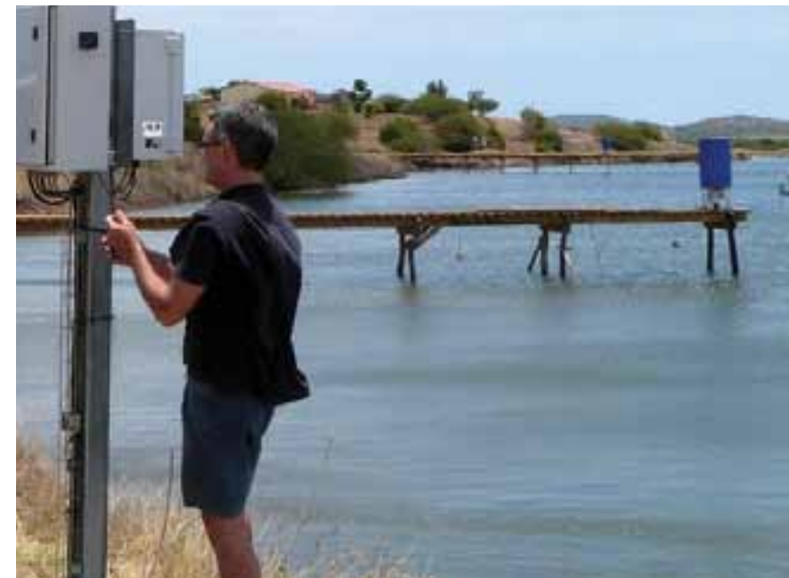
The sound feeding system enables sensor-based control of multiple feeders within ponds.
