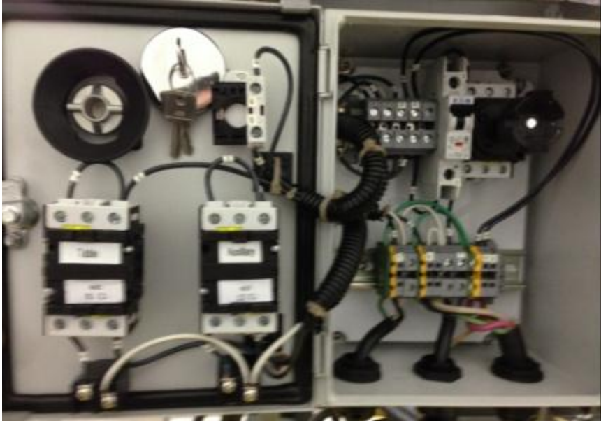
Figure 59 : Completed Control Box Interior
