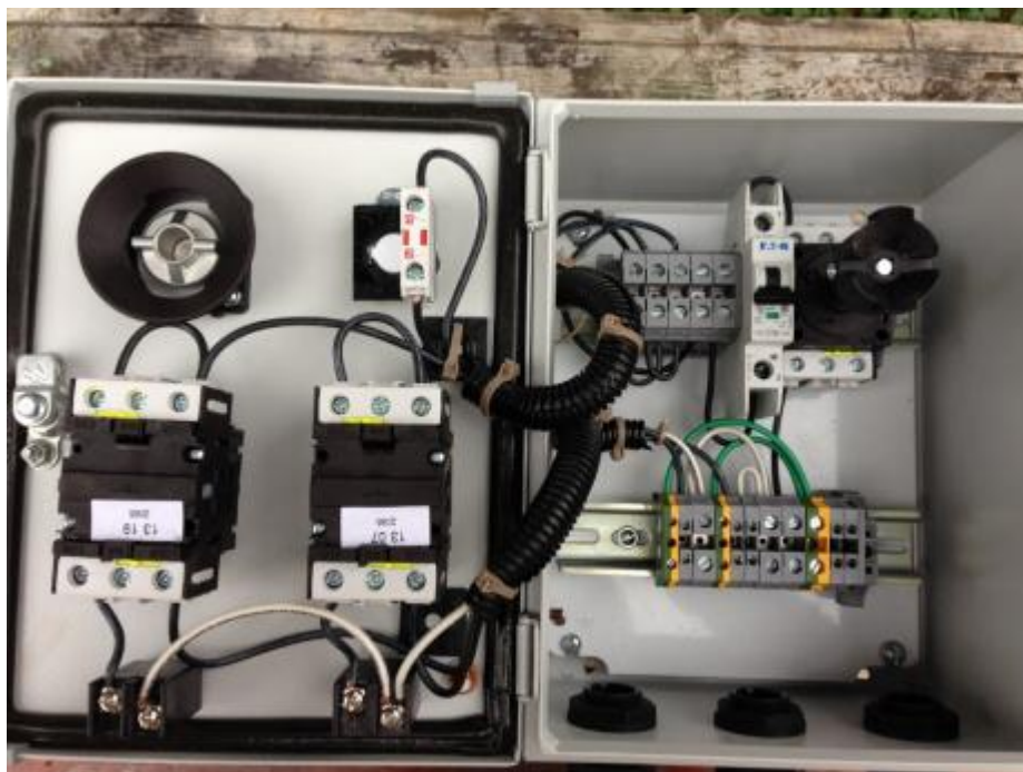
Figure 58 : Nearly Complete Control Panel
