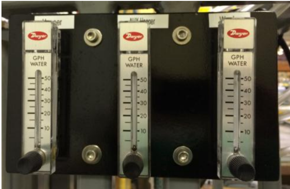
Figure 41: Flow Meters that Supply the Mixing Basin, Feed Basin, and Wash Box
