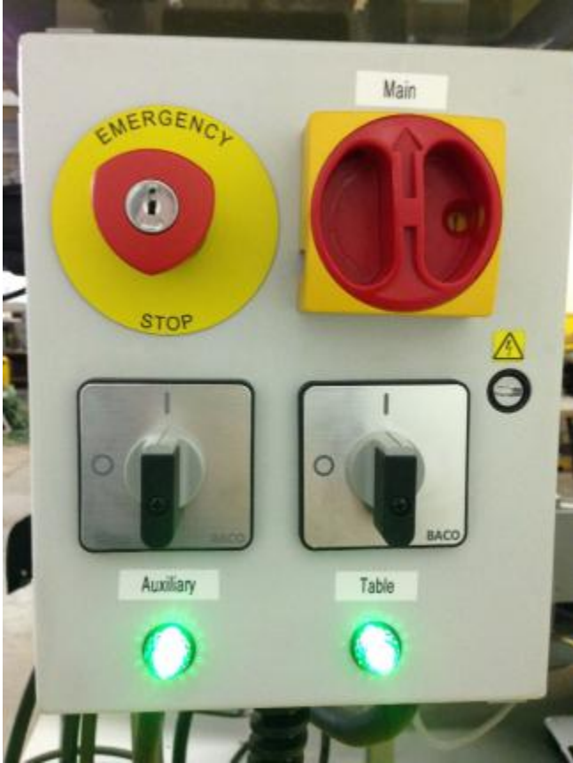
Figure 60 : Completed Control Box Exterior
