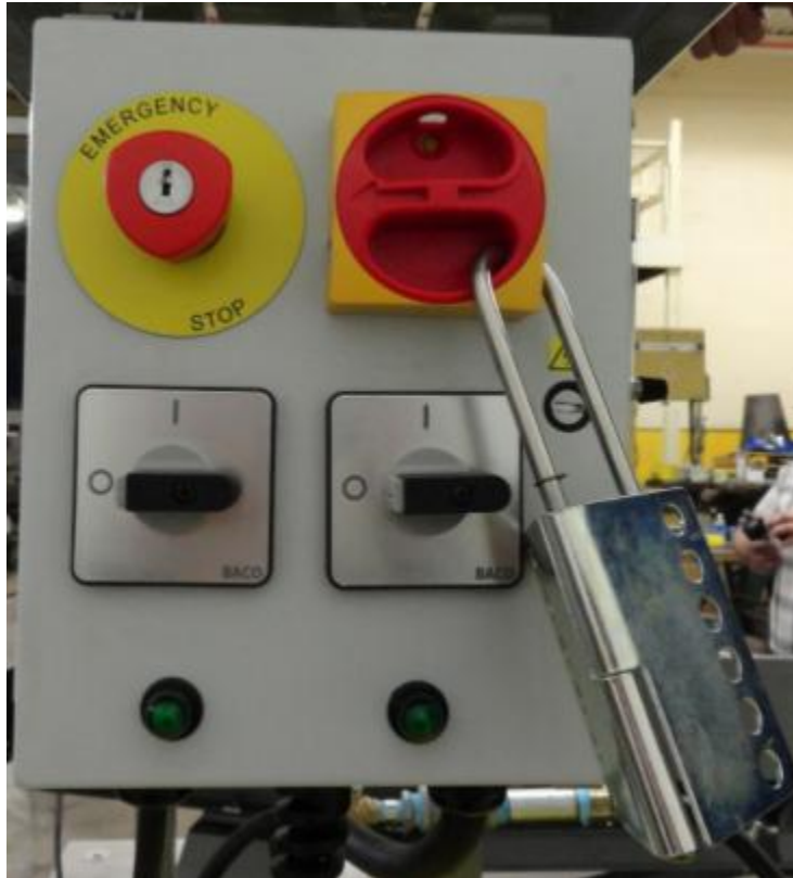
Figure 67: Emergency Stop and Locked out Main Switch
