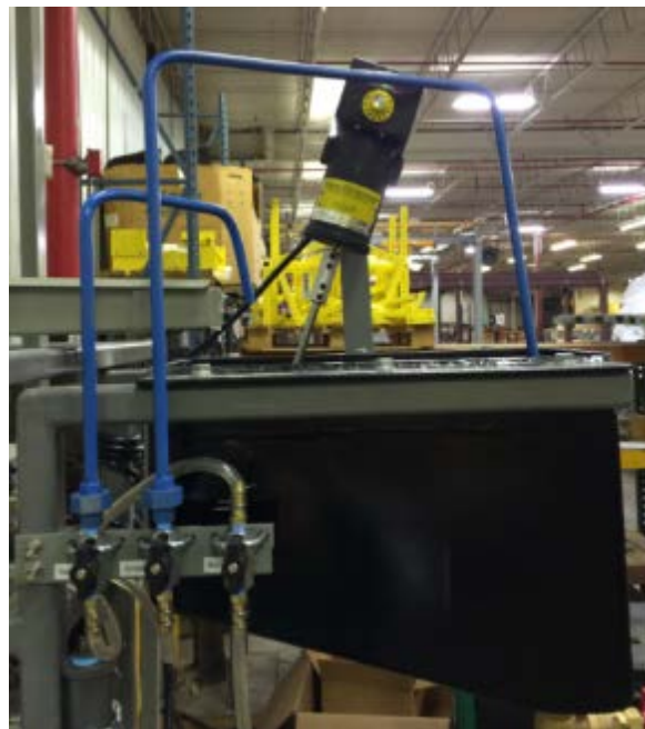
Figure 43: Shut-off Valves and Supply Lines to Mixing Basin and Feed Basins of the Hopper
