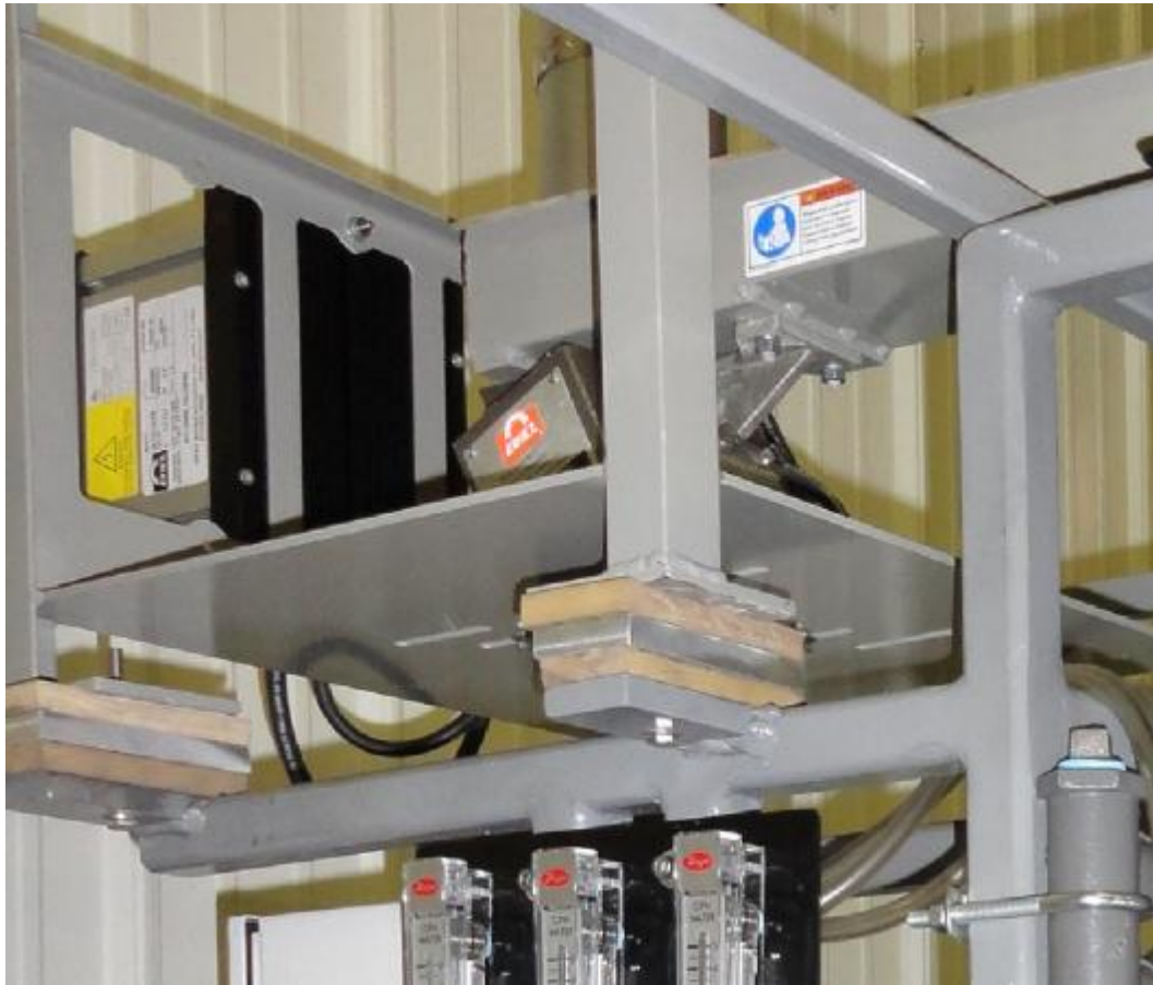
Figure 29: This Picture Shows the Vibration Mounts Used to Secure the Vibratory Feeder
