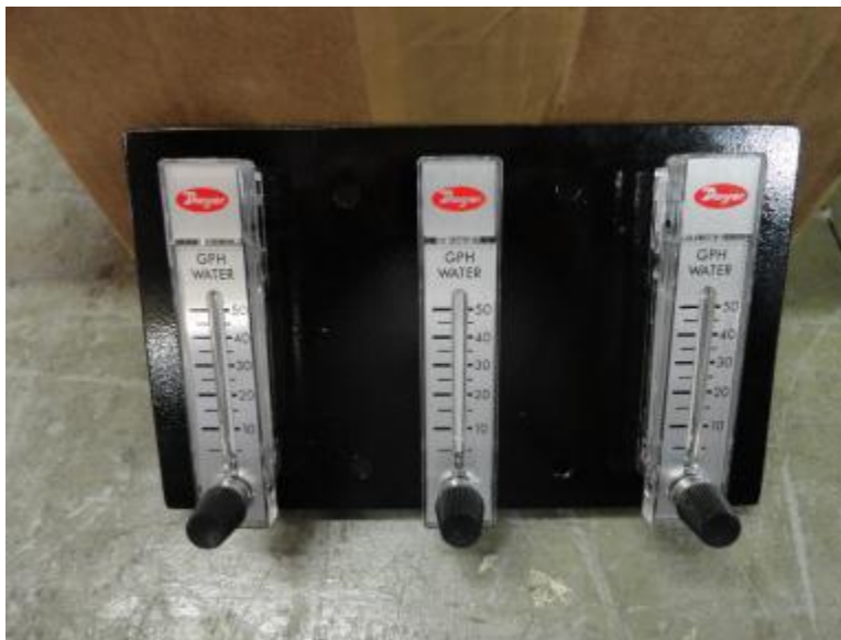
Figure 20: Finished Water Flow Meter
