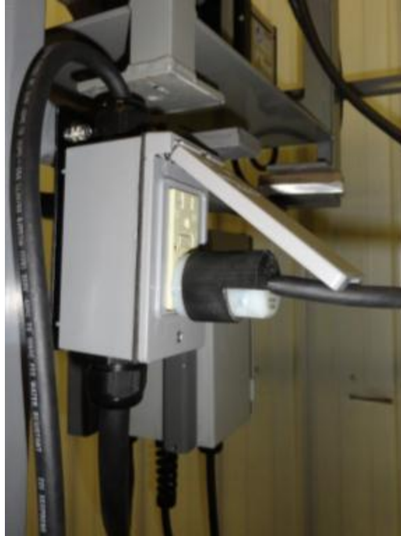
Figure 21: Finished Electrical Outlet Plate
