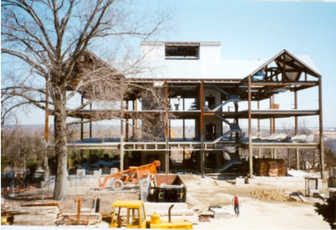
Figure 105. With just steel frame of Olin Science Center in place, the basic arrangement of corner towers and central service core is plainly visible. Photograph by Brian Rogers, 1994.
