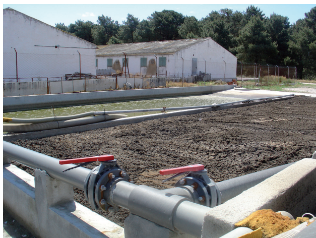
Figure 6.7.1. Coagulation/Flocculation unit of the treatment plant in Cuellar (Castilla y León, Spain).
