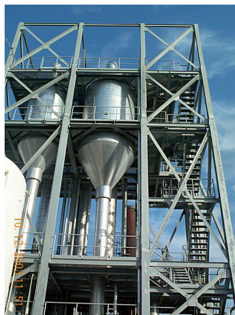
Figure 5.6.2. Vacuum evaporator. Tracjusa treatment plant (Catalonia, Spain)
