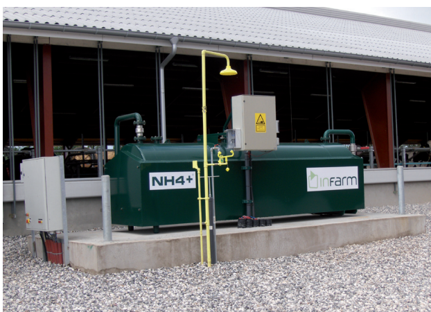
Figure 5.1.2. Infarm acidification unit ©Infarm
