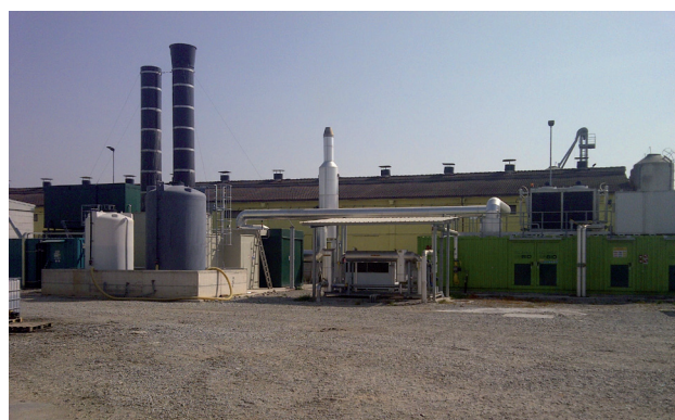
Figure 5.7.2. Dryer plant with scrubber and CHP. Green Energy farm - Brescia, Italy (CRPA, 2015).
