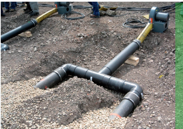
Figure 5.5.5. Windrow composting: static pile system with forced aeration. View of the air forced system.
