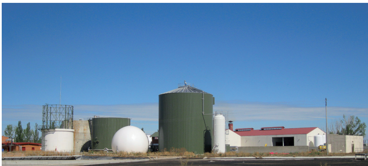
Figure 6.2.1. General view of the anaerobic digestion treatment plant in Almazán (Castilla y León, Spain).
