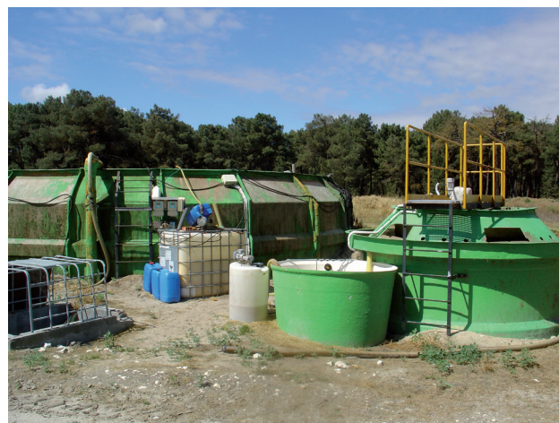
Figure 6.7.2. Aerobic biological treatment + settling of the treatment plant in Cuellar (Castilla y León, Spain).
