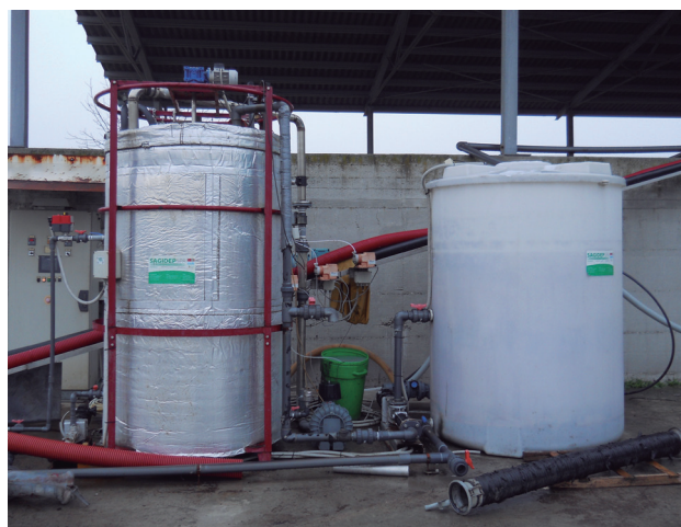
Figure 6.5.2. SHARON-SBR reactor in Campo Bò (Emilia Romagna, Italy).
