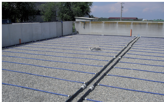
Figure 5.10.4. Plant developments in a H-SSF constructed wetland (CRPA, 2006).
