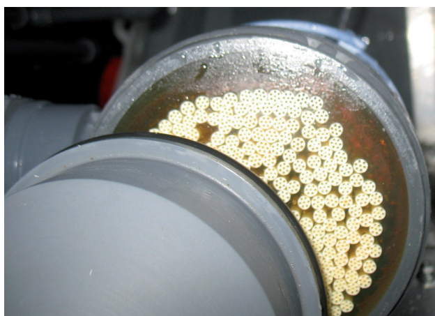
Figure 5.9.2. Ultra filtration unit.
