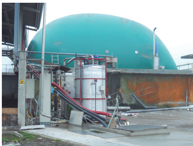
Figure 6.5.1. Anaerobic digestion, CSTR reactor and gasometer in Campo Bò (Emilia Romagna, Italy).
