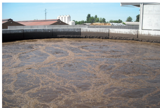
Figure 5.4.4. Aerobic process with aeration (left) and anoxic phase (right) in different tanks. In the foreground the sedimentation tank.
