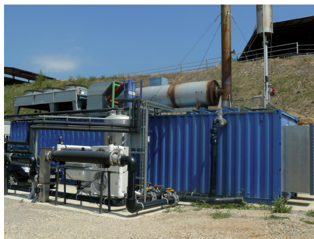
Figure 5.3.4. CHP engine fuelled by biogas
