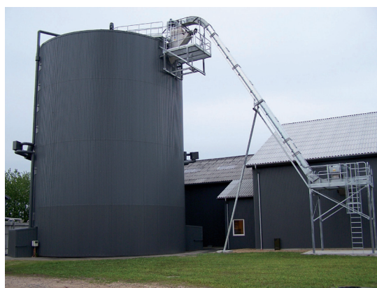
Figure 6.3.2. The main reactor with the new solids loading belt/screw system.
