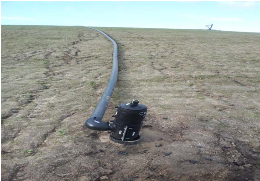
Figure 4.3: Gas collection pipe at landfill A (Author, 2013)
