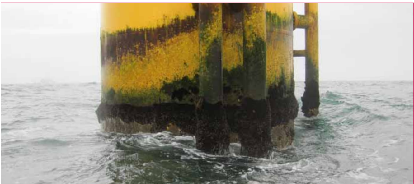
Concrete gravity based (upper panel) and steel monopile (lower panel) foundations on the Thorntonbank and Bligh Bank, respectively
