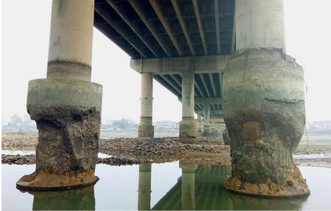
Figure.4 Voids and hungry spots on bridge piers (Voids on Lishui River Bridge, 2016)
