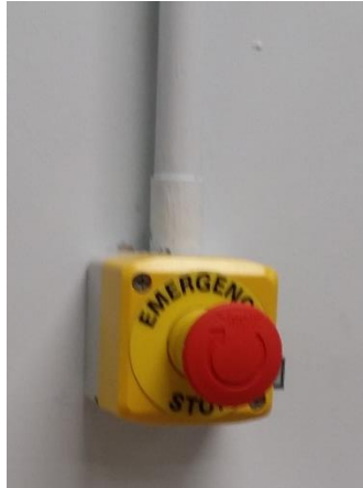
Figure F-8 Emergency Stop Switch
