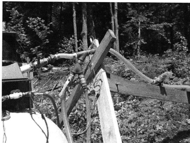
Figure 57: A wooden structure provides support for the valve assembly.
