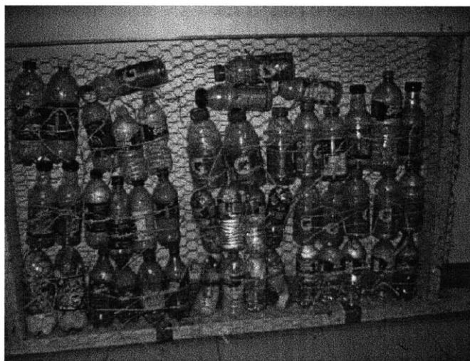
Figure 6: A 4 feet by 2.5 feet section of wall was built to gain knowledge from the process of building the wall.
