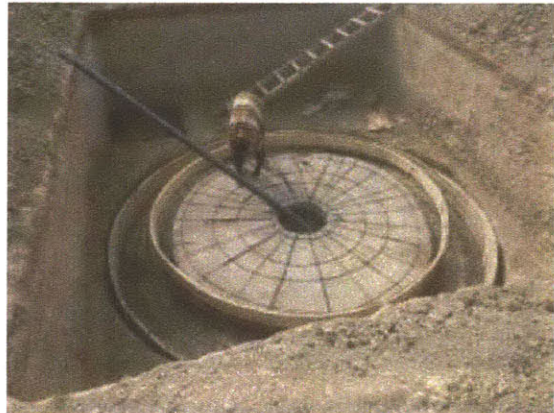
Figure 25: The steel bender links reinforcement for tank floor with reinforcement for footing
