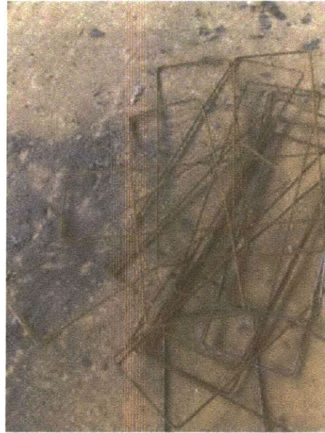
Figure 21: Close up of rectangular pieces that binds concentric circles of rebar together for the footing
