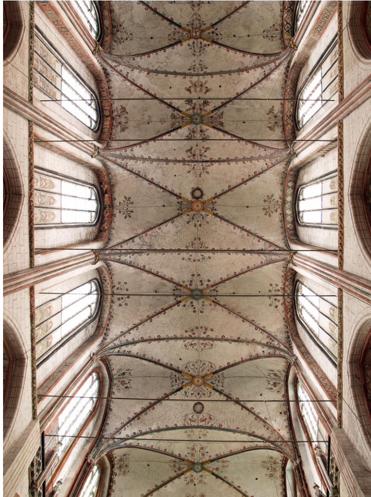
Figure 3.3: As in the main nave of St. Mary's church in Lübeck the brick groin vault has a distinct structure, defined by its geometry, and a distinct material (bricks). Being constructed from only one material however, the groin's structural stability is achieved by its geometrical arrangement. In the case where the point of failure occurs between neighboring bricks, one may refer to the material as the structural unit. Failure is defined by the size hierarchy at which the main interfacial influences occur.
