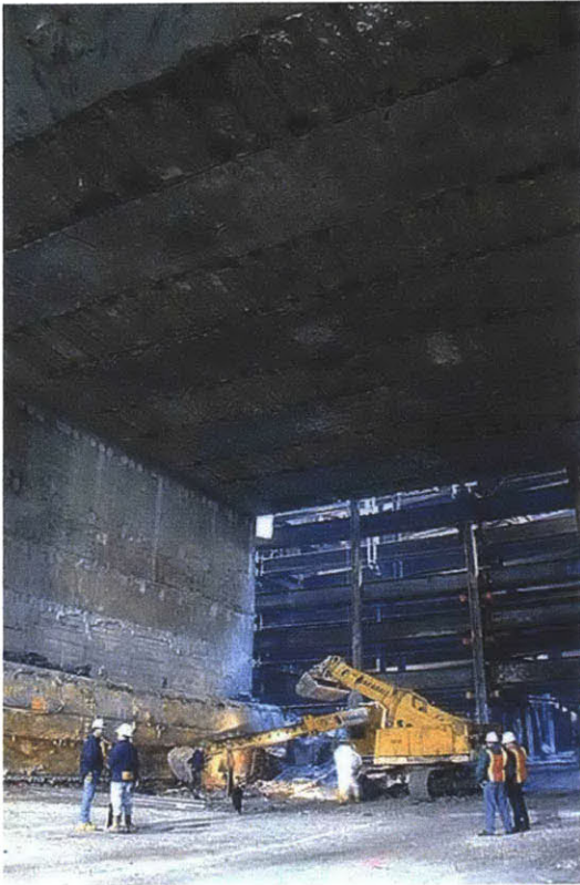
Figure 29 Underpinning structure below the Red line subway, fully excavated and ready for construction of the highway [12]
