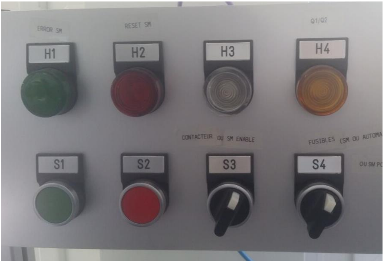
Figure 15 : Rack 4 lights et 2 switches
