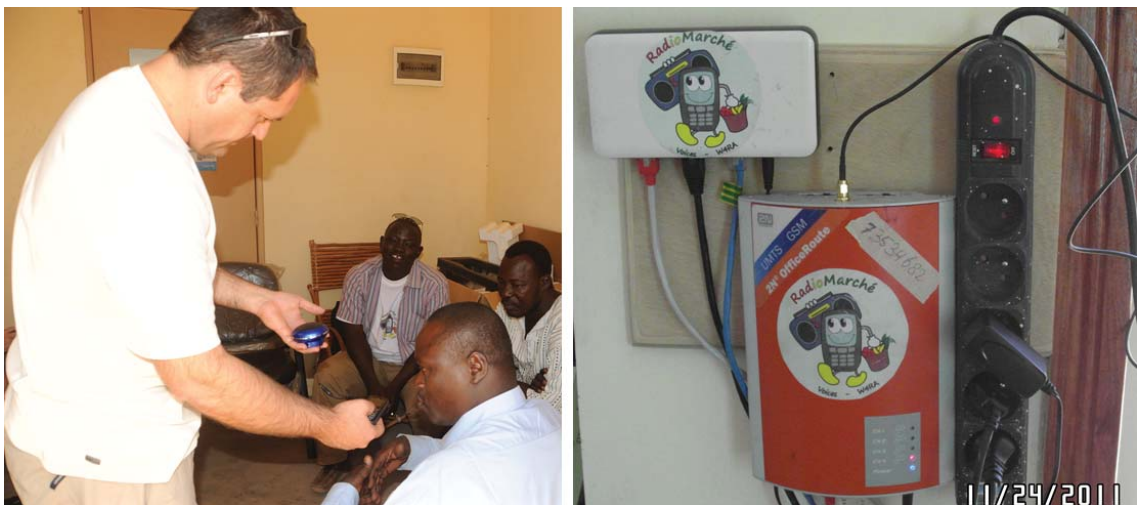
Figure 4.9: Implementation of the RadioMarché system in Mali. On the left, an audio recording and evaluation session needed for building the TTS engine is shown. The right part of the image shows the OfficeRoute GSM gateway which is part of the local standalone installation of the hardware setup.
