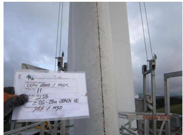
Figure 3 Front edge cracks (transverse and longitudinal)
