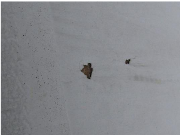
Figure 6 flaking of the top coat
