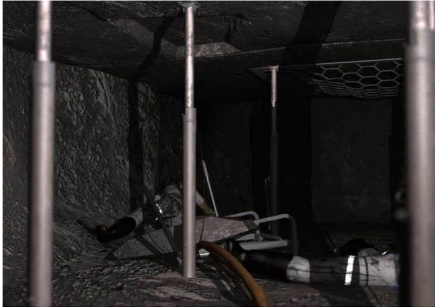
Figure 2.8D: Workers injured due to a rock fall.
