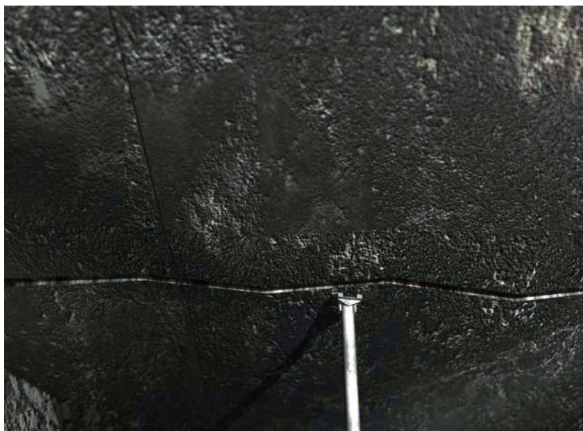
Figure 2.8A: Workers identified a number of intersecting joints.
