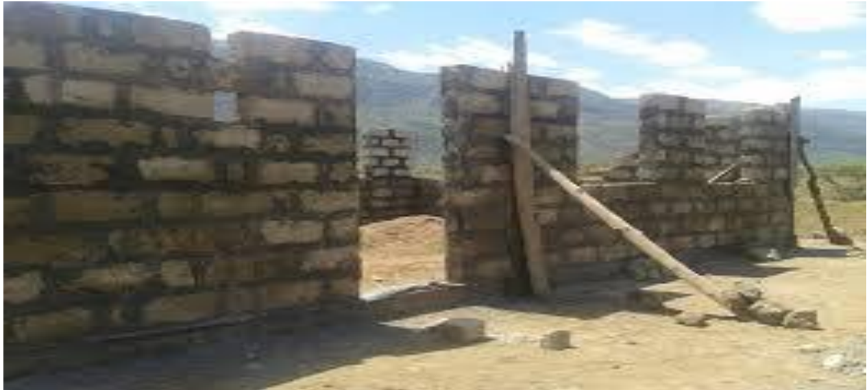
Figure 11: Incomplete construction of classrooms at Kimotorok Primary School.
