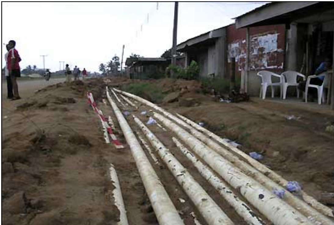
Fig. 4.18 Pix showing ruptured water pipes in Niger Delta. (Field study, 2009).
