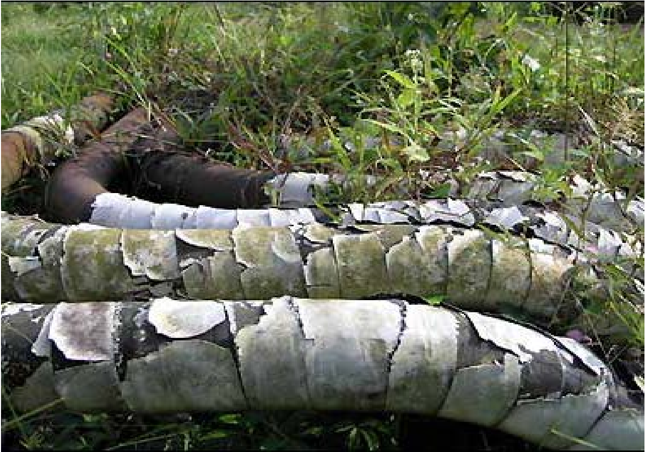
Fig. 4.20 Pix showing Ruptured high pressure oil pipe. (Field trip June 2009).
