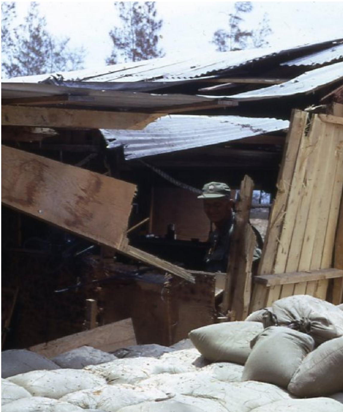
Figure 16. Artillery Damage to Cua Viet Barracks. Captain Shaw, Commander of Task Force Clearwater, inspects damage to his office, March-April 1968. Photo courtesy of Herman Hughes.
