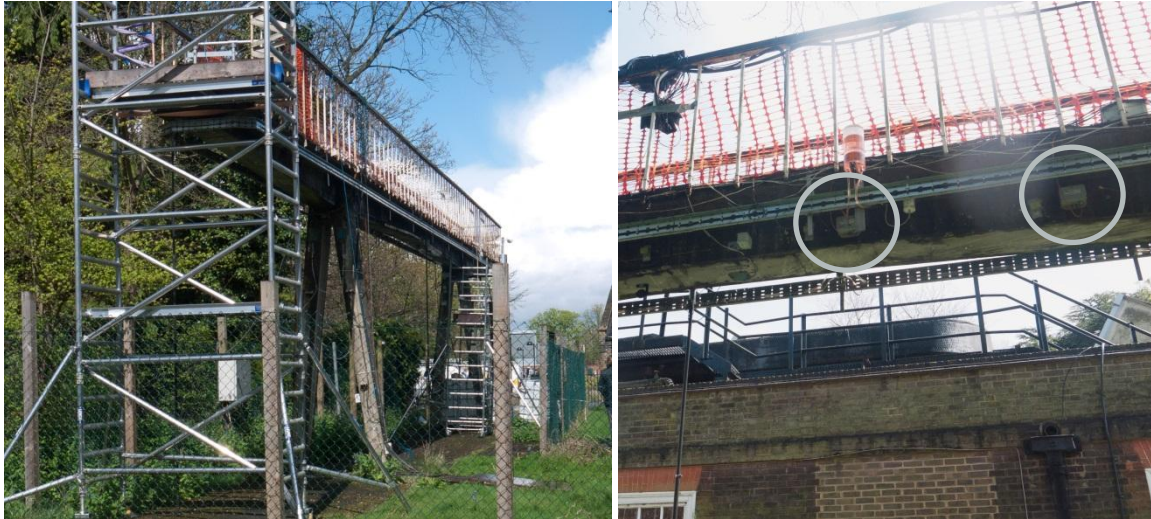
Figure 7: Front view of the NPL footbridge (left) and back view of mid-section of the footbridge (right) and a tilt-meter (circled).
