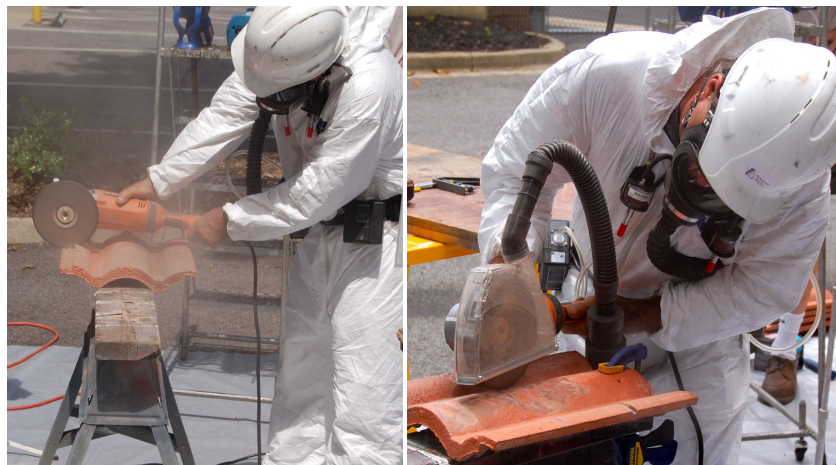
Figure 6.2. CPWR demonstrates the effectiveness of ventilation with construction nanomaterials. Here, a worker using a tile cutter on a clay roofing tile and producing a large amount of clay dust (on the left) can control exposure using a fitted vacuum hood (on the right). (Images courtesy of B. Lippy.)
