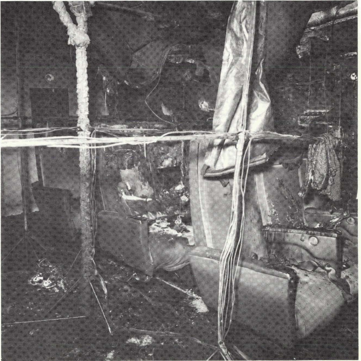
Figure 16.- Fire damage for test 1 using pre-1968 materials, front view.
