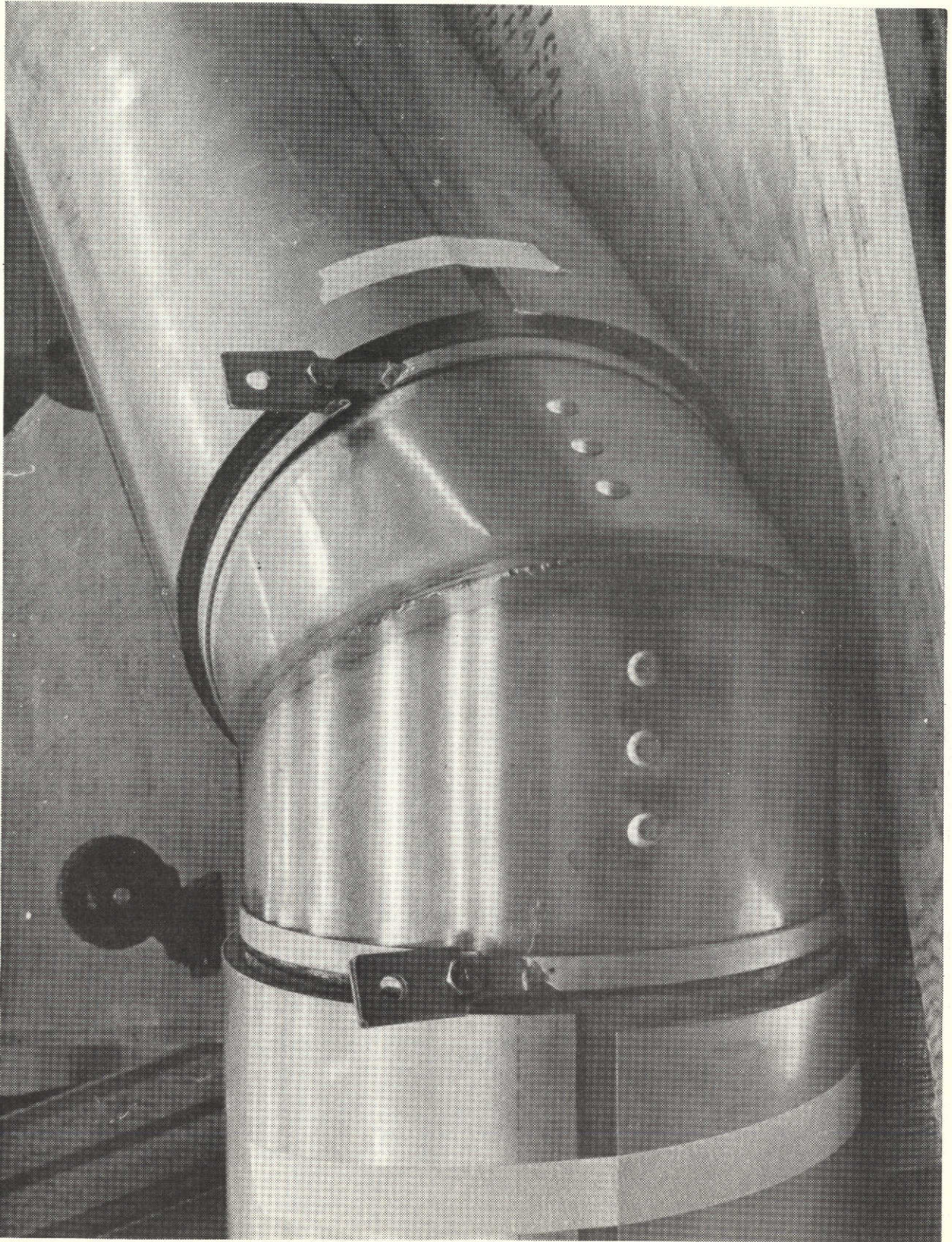
Figure G-1. Elbow Zone Details Showing Rivets and Support Clamps
