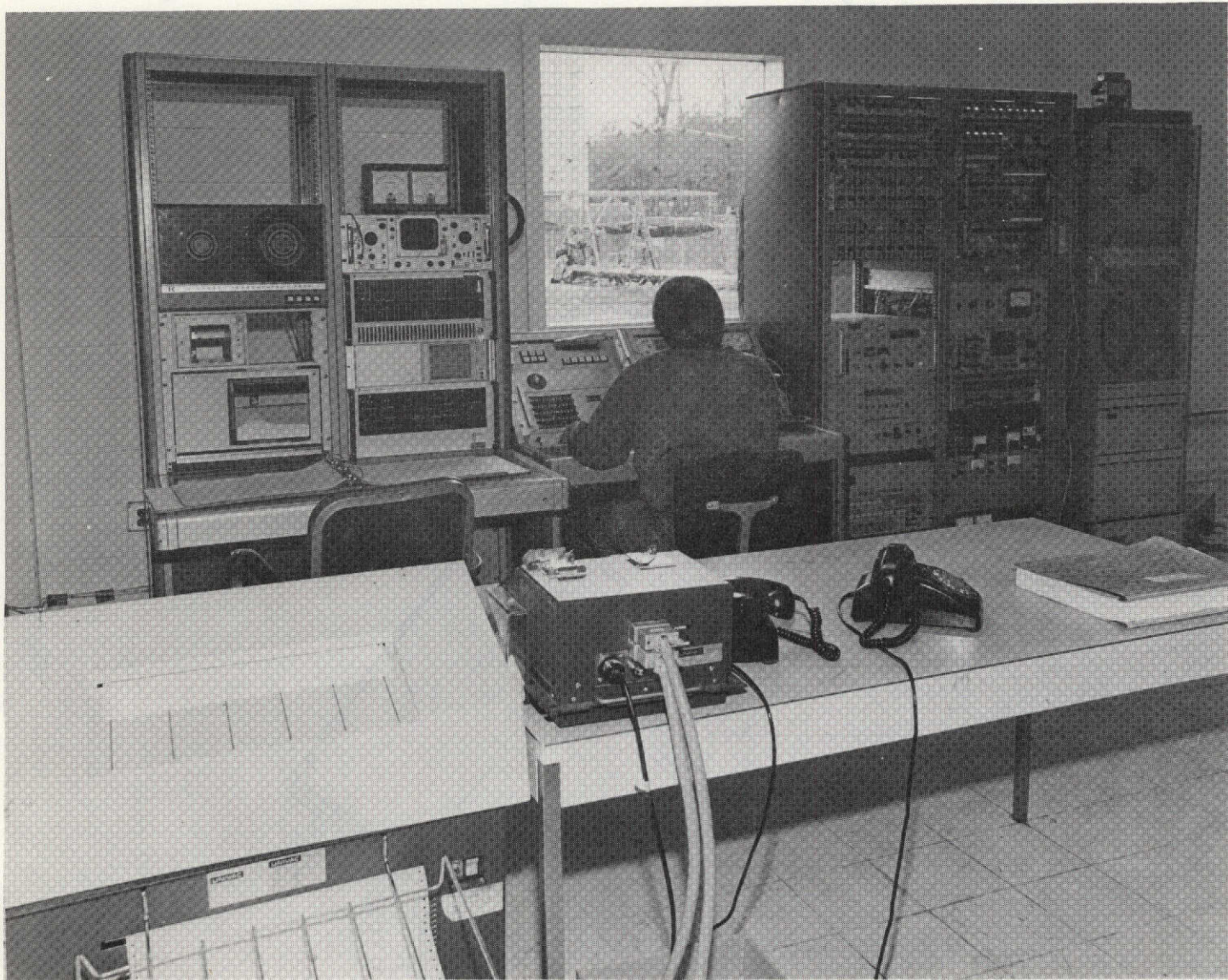
Figure 15 View of data acquisition system.
