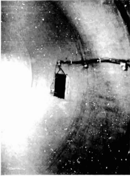
HEAT FLUX GAUGE (HF2) AND TEMPERATURE SENSOR
