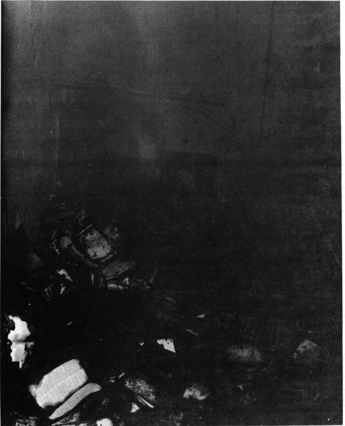
FIGURE 9. "TYPICAL" ROOM AFTER FIRE
