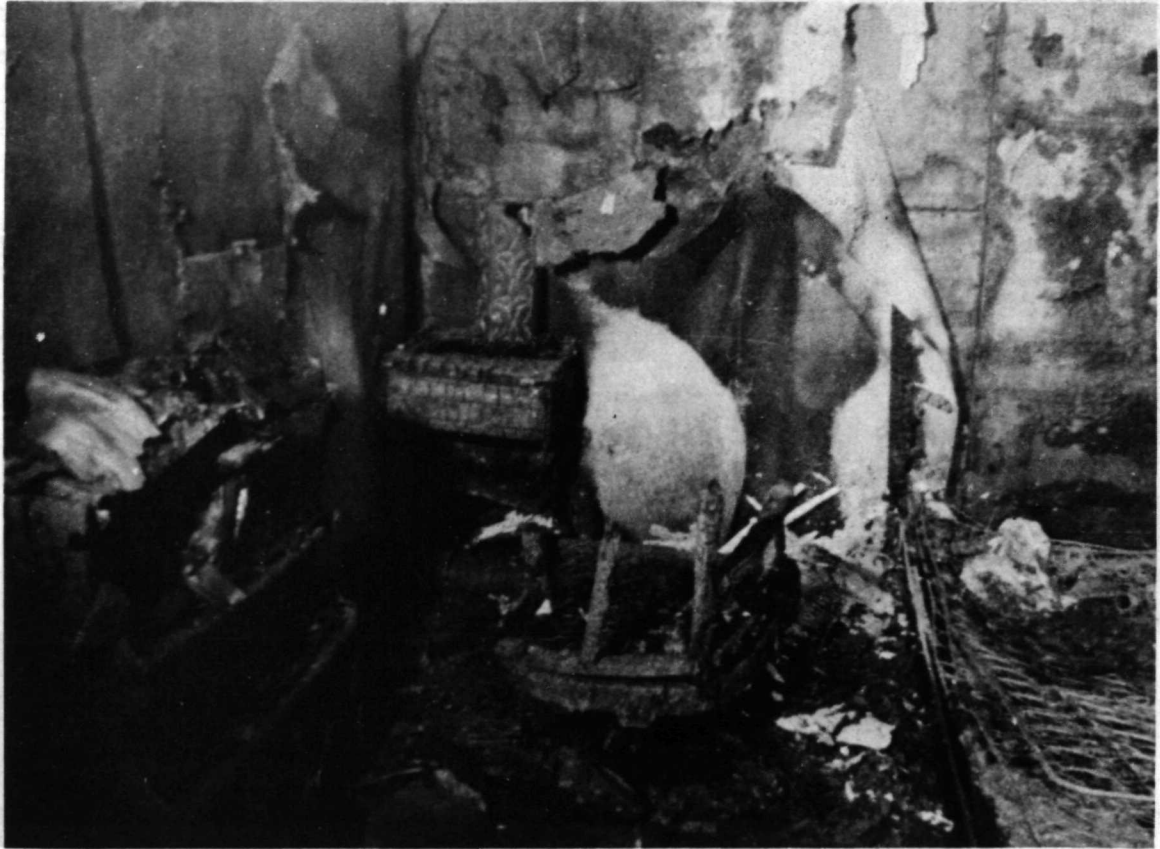
FIGURE 11. "IMPROVED" ROOM AFTER FIRE
