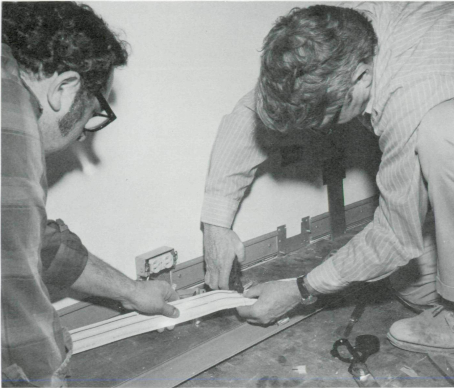
Baseboard installation of flat conductor cable by the Urban Development Corporation in garden apartment units in Yonkers, New York.
