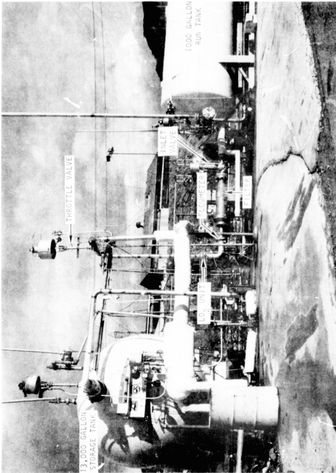
Figure 46. LO 2 Flow Facility With LO 2 Unit No. 1 Installed
