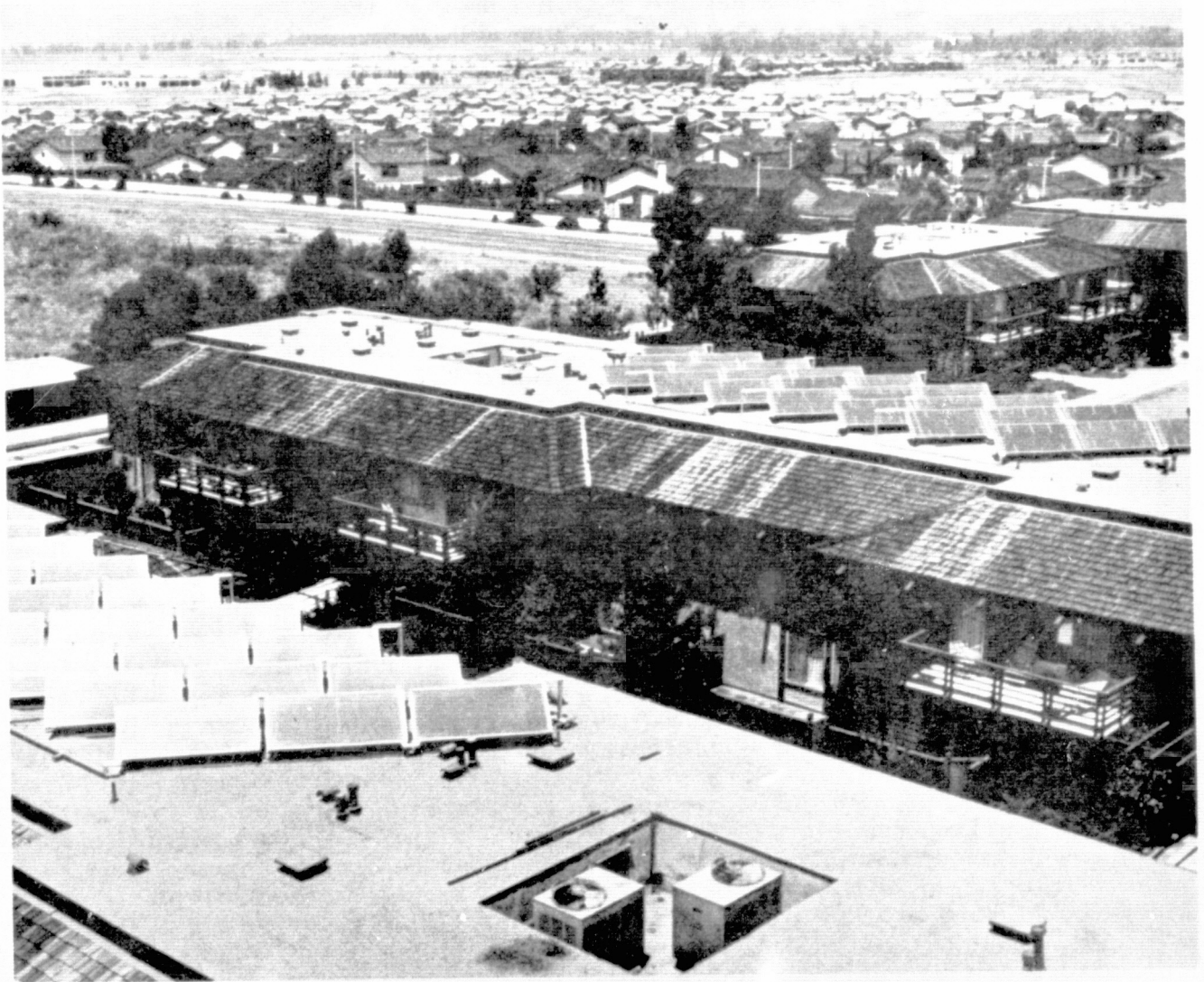
Figure ES-1. SAGE Active Solar Energy System on an Apartment Building in Southern California
