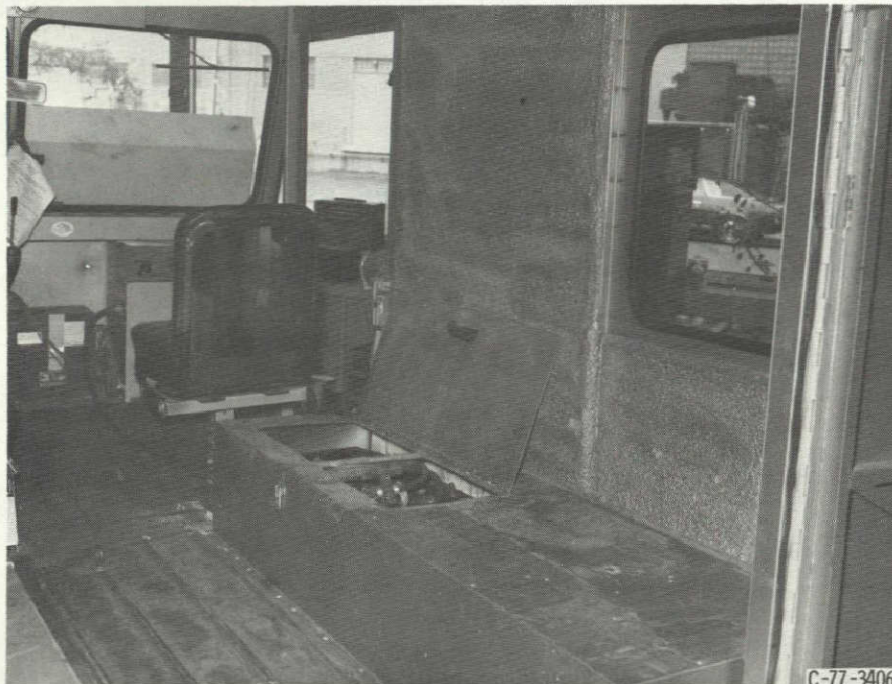
Figure 4. - View through rear door showing right battery pack. Charger is immediately in front of passenger seat.
